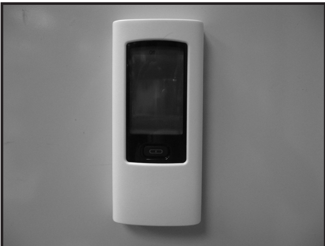
Figure 3.10 Mounted Remote Control Housing
